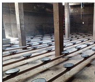
Figure 1: fine bubble diffuser mesh inside aeration tank
