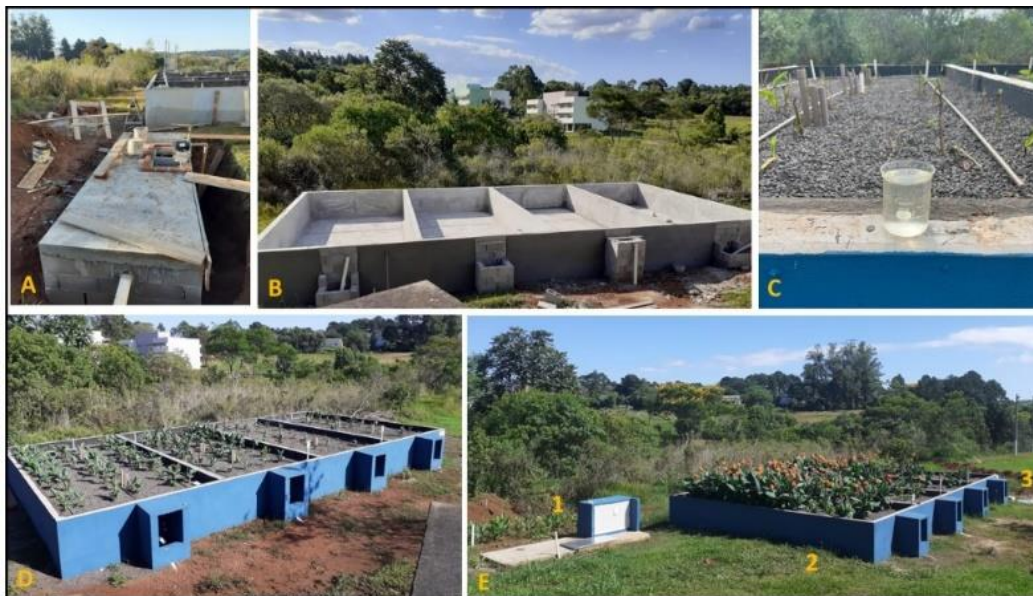
Figure 1. Decentralized wastewater treatment plant: Construction (A-B) and Operation (C – after 30 days; D – after 90 days; E – after 120 days) 1. Septic Tank and Pump Station; 2. VFCW; 3. UV unit.
