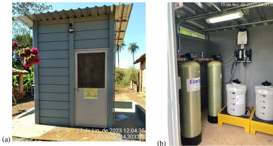
Figure 1 – Treatment system implemented, comprising (a) cover and (b) water filtration unit
