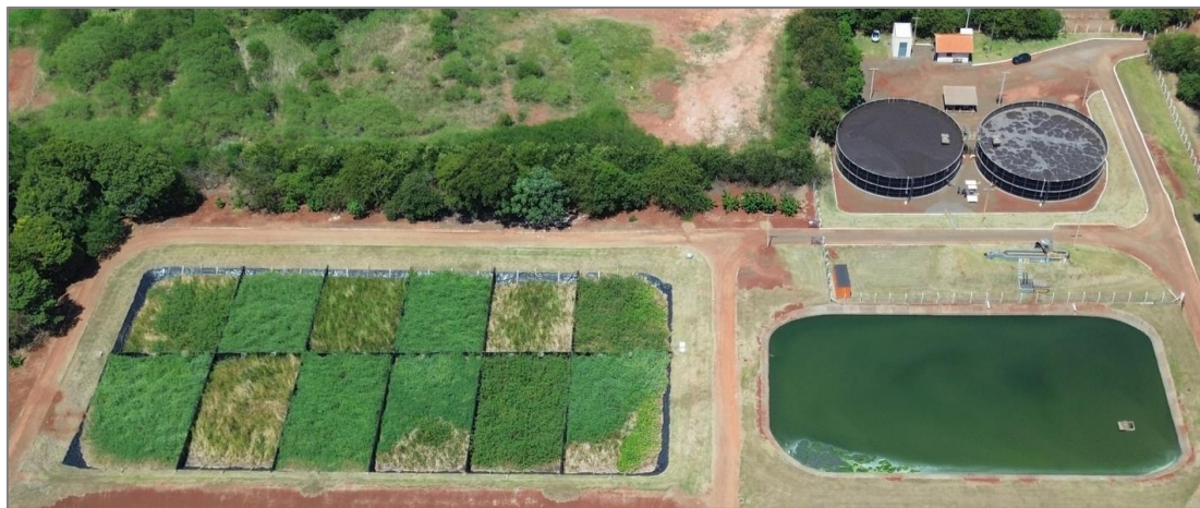
Figure 1: Aerial view of Santa Helena WWTP showing 2 SBR reactors and Sludge Treatment Wetlands divided into 12 separate beds, installed in the former maturation pond.
