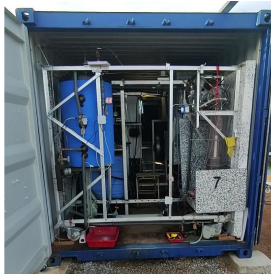
Figure 1: System (containerized) used during the tests in the city of Quixeramobim, Ceará state, Brazil.
